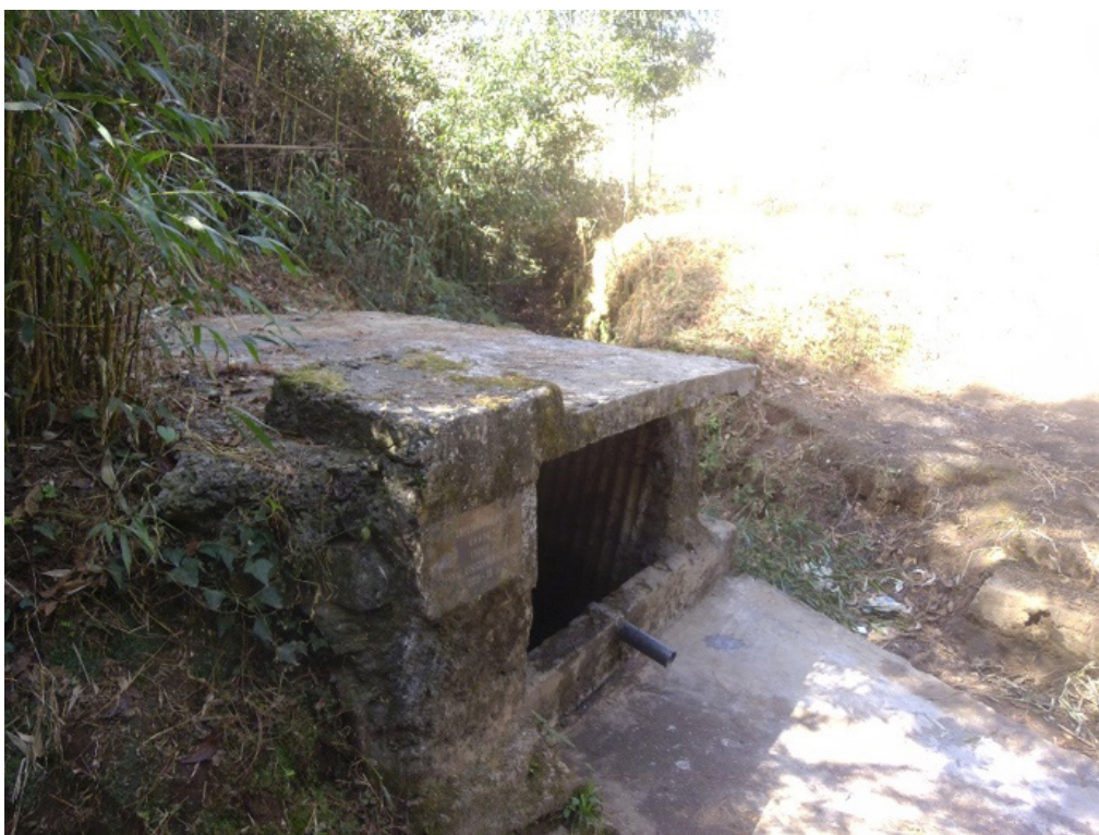
Fig. 24: A concrete well for storing spring water
